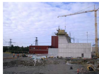
Side view of converter transformer bunker (Rauma), existing pole in background
